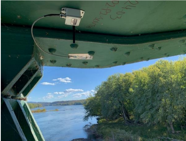
Strain SenSpot sensor in girder for fracture critical monitoring
