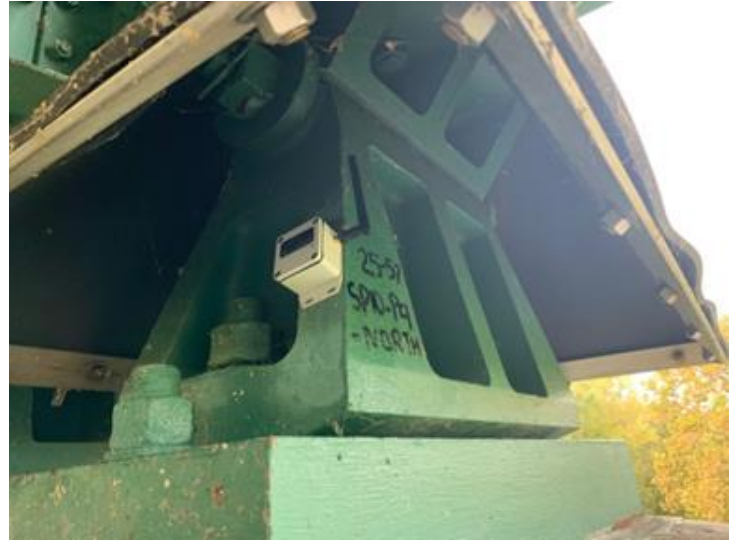
Tilt SenSpot sensor on bearing for bridge fracture critical monitoring
