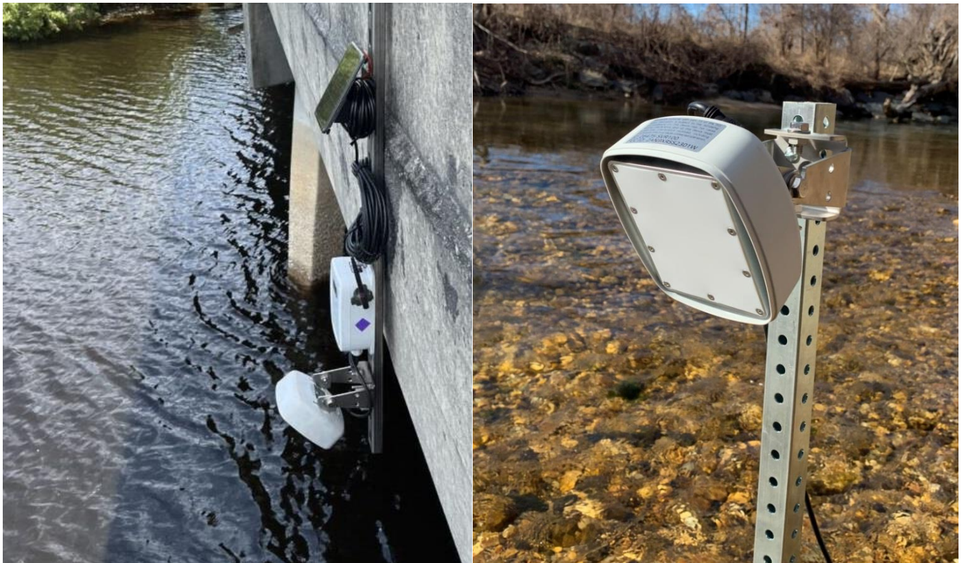
Figure 3: An installed Resensys wireless water velocity SenSpot™ .
