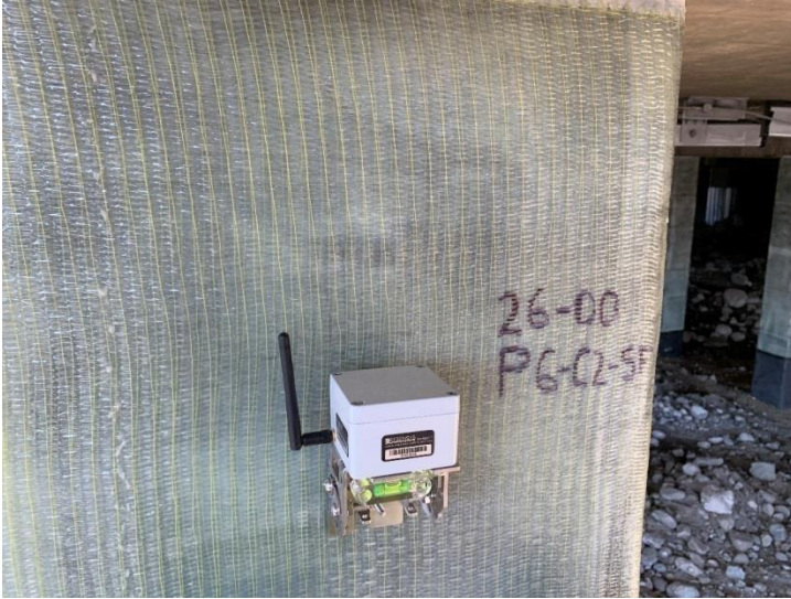
Resensys Wireless Tilt/Inclination SenSpot™ sensor on pier for monitoring bridge under superloads
