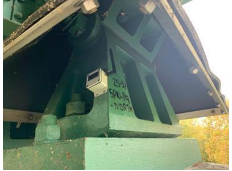
Resensys Wireless Tilt SenSpot™ sensor on bearing for monitoring bridge under superloads
