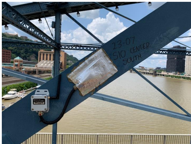
Figure 1: Wireless strain gauge SenSpot™ at a truss of a bridge
