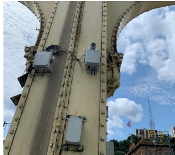
Figure 2: Resensys wireless solar powered camera installed on the pier of a bridge to provide complete visual feedbacks of overweight loads
