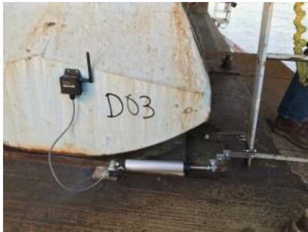
Resensys Wireless Displacement SenSpot sensor on bridge bearing to assess bearing functionality
