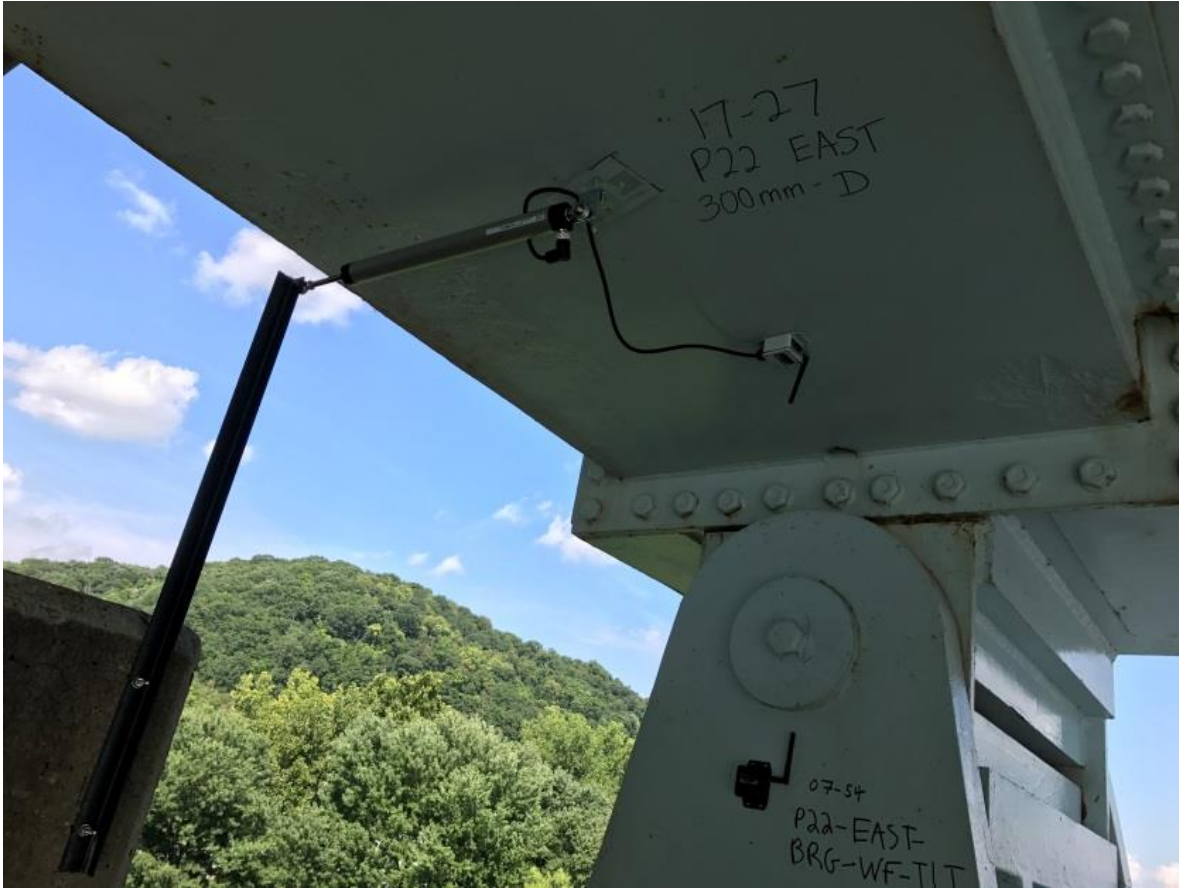
Tilt (bearing rotation) SenSpot sensor and displacement SenSpot sensor on bridge bearing to assess bearing functionality
