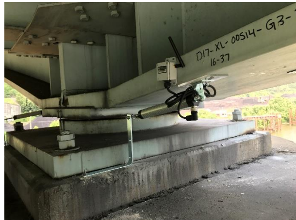
Resensys Wireless Displacement SenSpot sensor on a bridge expansion joint
