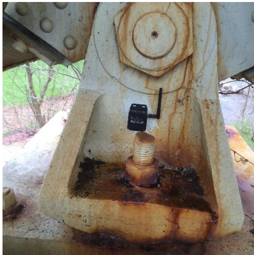
Resensys Wireless Tilt SenSpot sensor on a bridge bearing to assess bearing functionality
