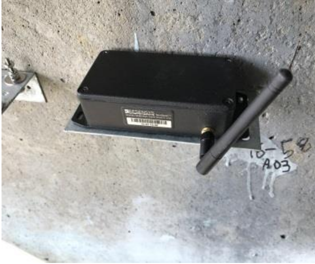
Resensys Wireless Vibration/Acceleration SenSpot™ sensor on pier of a bridge for measuring pier acceleration and barge collision detection and monitoring
