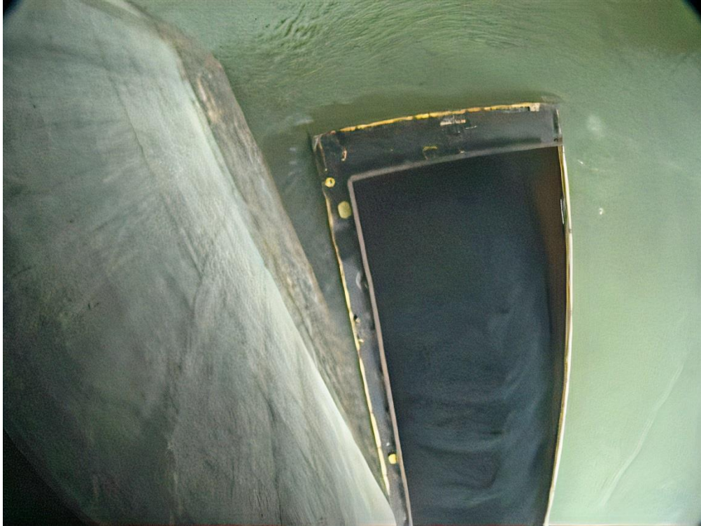
A typical picture taken by Resensys Wireless Solar Powered Camera indicating the field of view when there is a barge floating in close proximity of the pier. (This kind of picture can be time-stamped).
