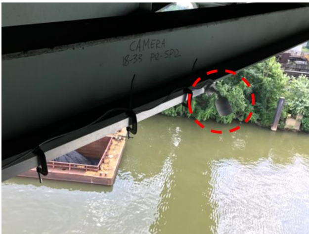
Resensys Wireless Solar Powered Camera on a bridge for barge collision detection and monitoring
