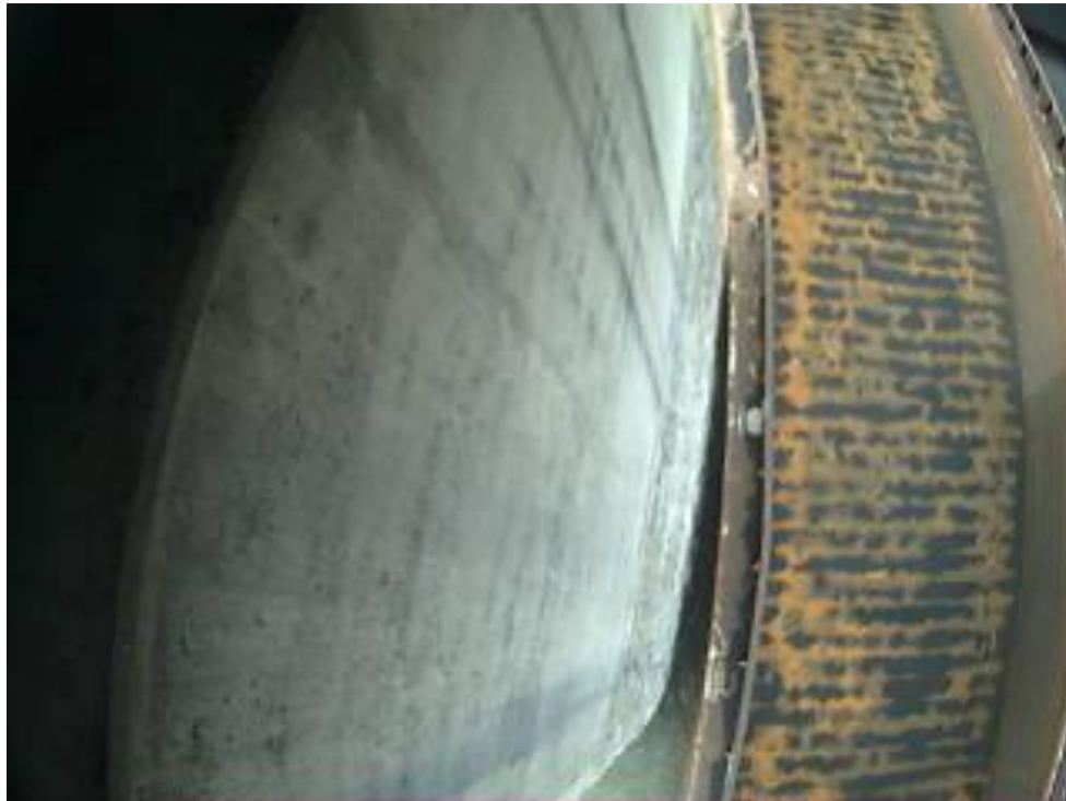
A typical picture taken by Resensys Wireless Solar Powered Camera that shows a barge at very small clearance of the bridge pier is passing (at the time of the detected impacts) (This kind of picture can be time-stamped)
