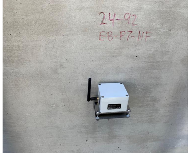
Resensys Wireless Tilt/Inclination SenSpot™ sensor on pier of a bridge for measuring pier rotation and barge collision detection and monitoring
