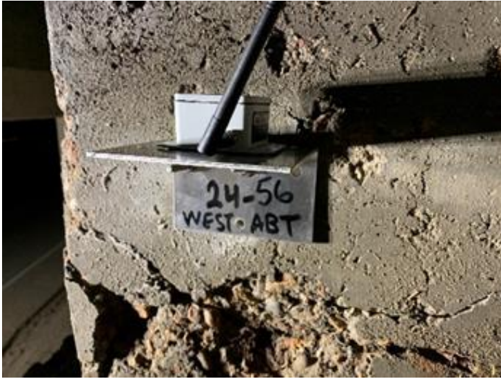
Vibration SenSpot™ sensor on a abutment for man-made seismic effect quantification/ vibration monitoring
