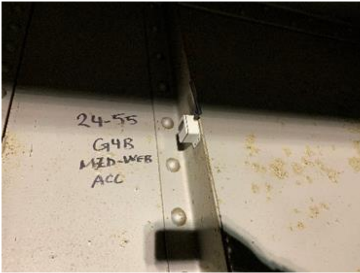
Vibration SenSpot™ sensor on the middle web of a span girder for man-made seismic effect quantification/ vibration monitoring
