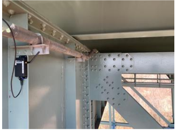
Vibration/ Acceleration SenSpot™ sensor on a abutment for man-made seismic effect quantification/ vibration monitoring
