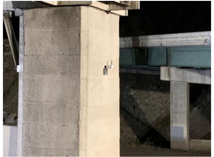
Vibration SenSpot™ sensor on a pier for man-made seismic effect quantification/ vibration monitoring
