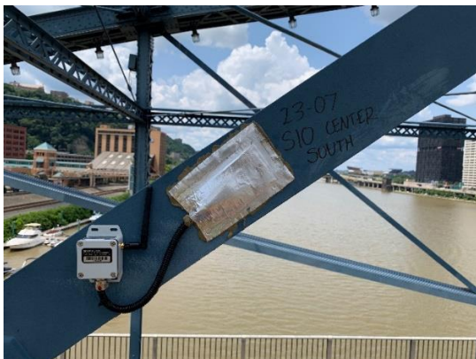
Wireless strain gauge SenSpot™ at a truss of a bridge
