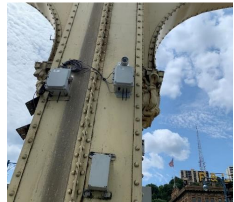
Resensys wireless solar powered camera installed on the pier of a bridge to provide complete visual feedbacks of overweight loads
