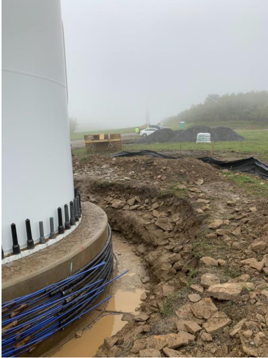
Monitoring turbine with Resensys wireless SenSpot™ sensors
