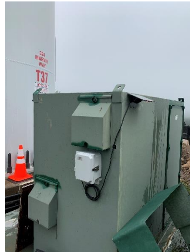
Solar Powered SeniMax™ Gateway installed for data acquisition
