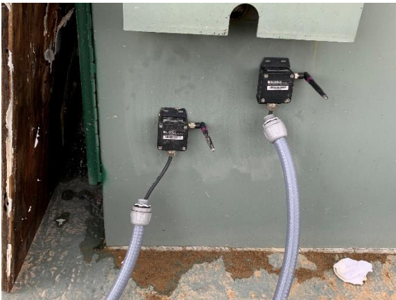
Wireless Strain gauge SenSpot™ for monitoring foundation of turbine
