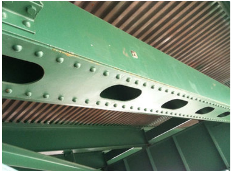
The sensors already are in place on the Northwest Branch Bridge in Silver Spring. (Courtesy Mehdi Kalantari/University of Maryland)
