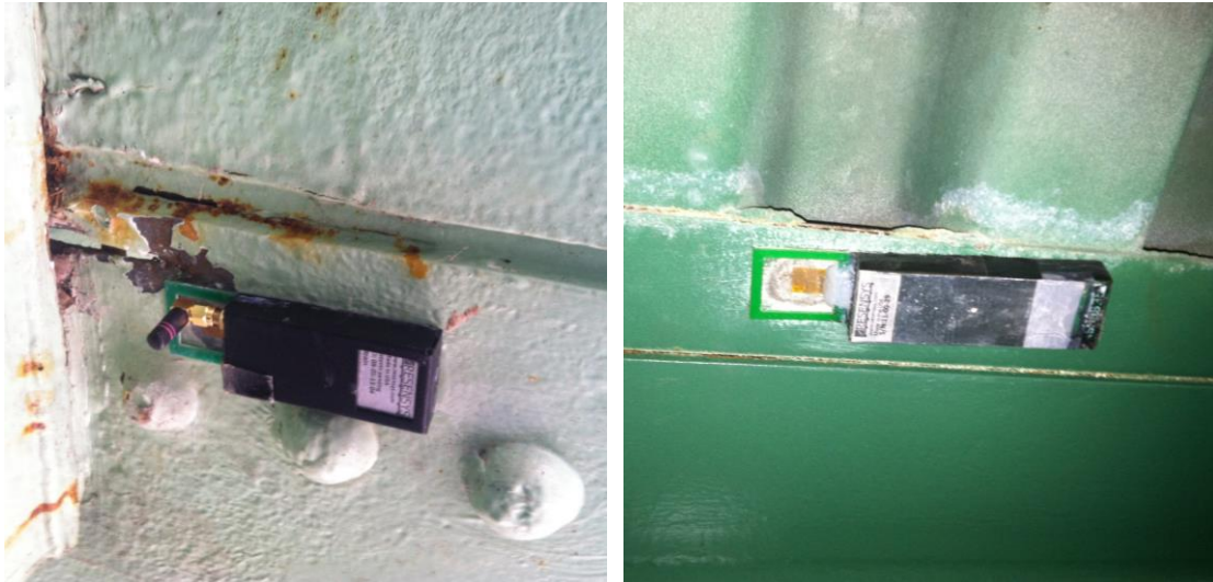
Figure 3: Strain gauge SenSpots installed on the bridge girders.
